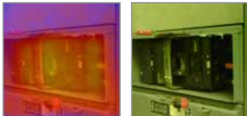
Normal operating temperature on mission critical breaker
